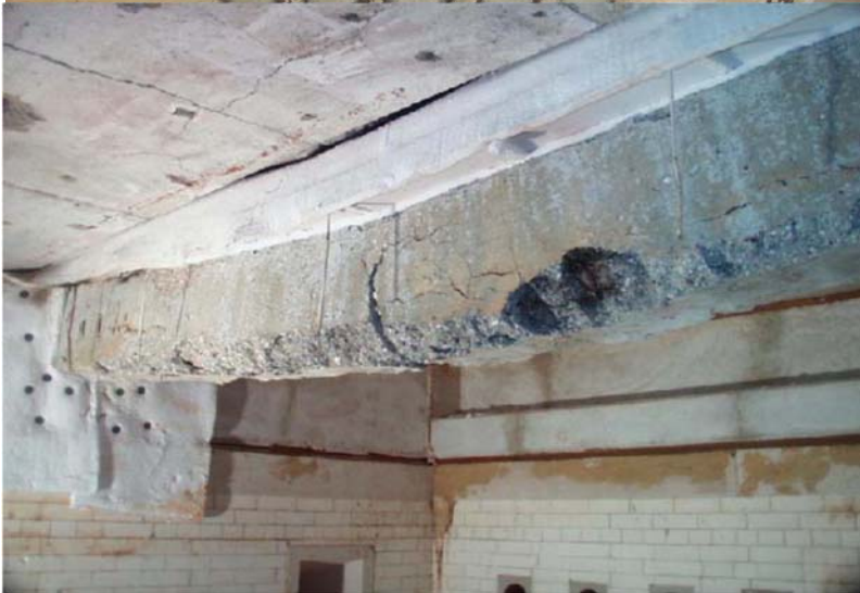
Figure 4. Beam after cracking
