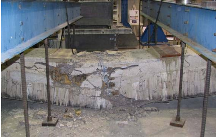
Figure 5. concrete beam flange cracking
