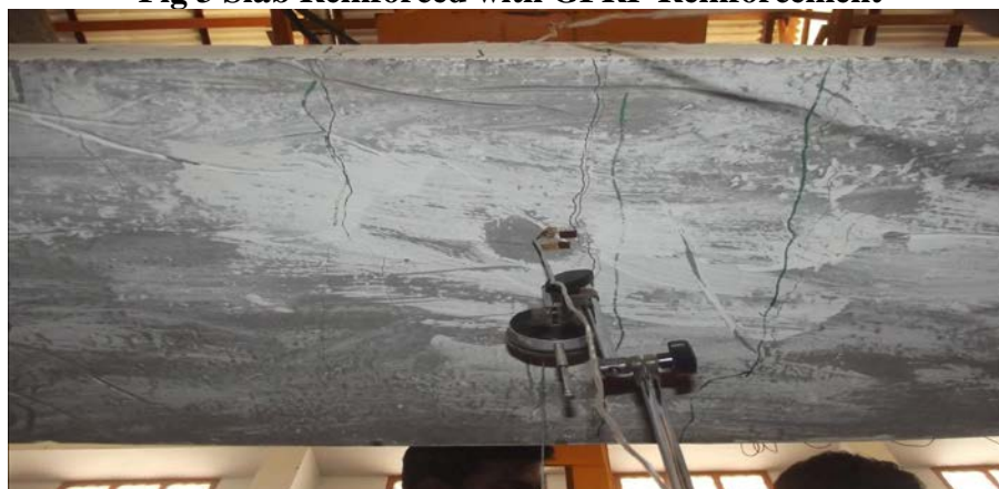
Fig 4 Crack Pattern for Conventional Concrete with GFRP
