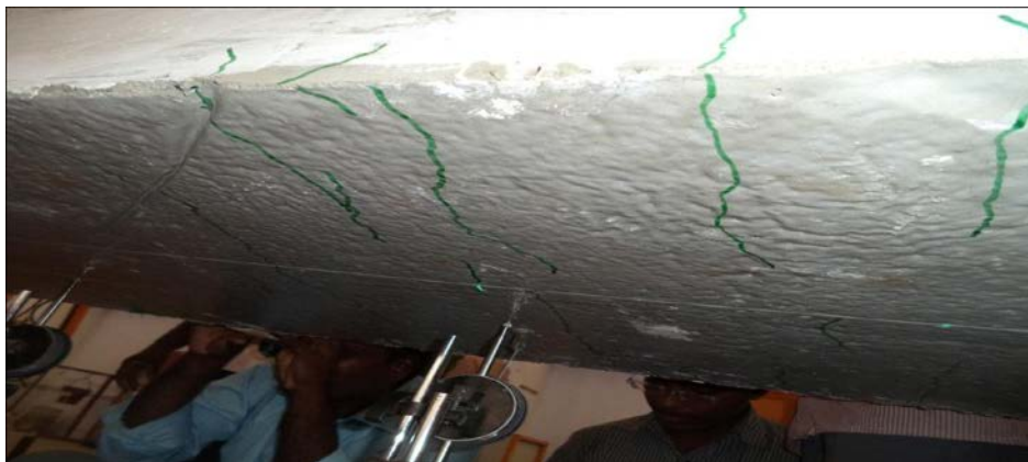
Fig 5 Crack Pattern for Geopolymer Concrete Slab with Steel Reinforcement
